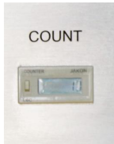
counter of booster pump
