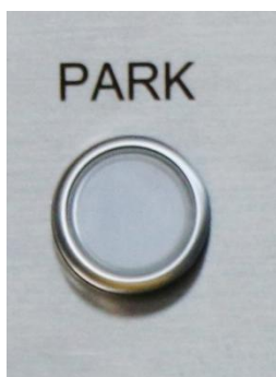
the working switch of booster pump
